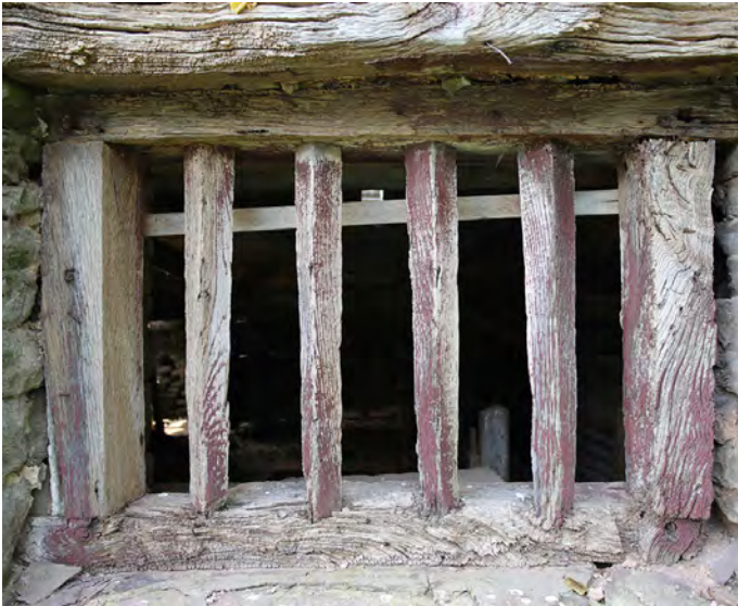
LEFT: Wood-mullioned windows of 18th century and earlier date are very rare. Photo © Sam Hale
