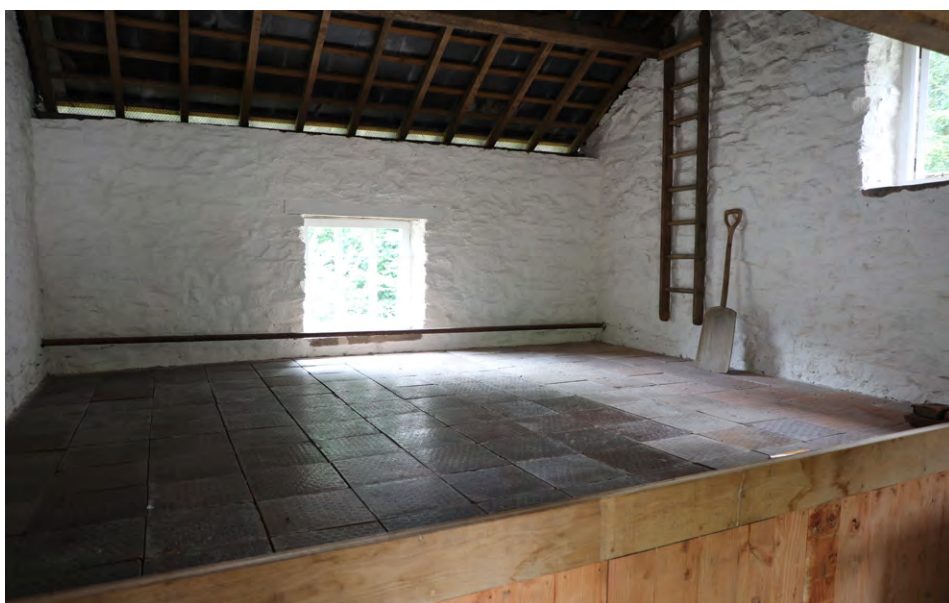
The 19th century two-storey drying-kiln abutted to the corn mill at Priory Mill, Brecon – the buildings and kiln floor altruistically restored by owners Noel and Susie Gaskell. Photos © Sam Hale
