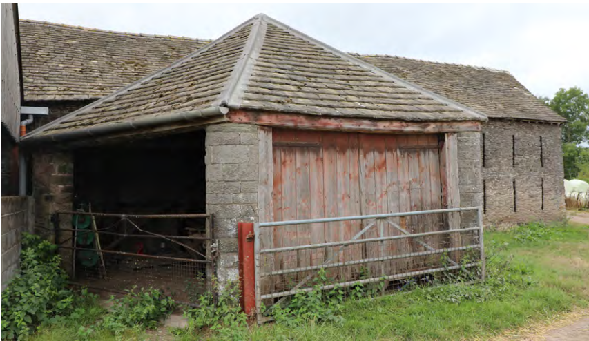
A rare surviving example of a horse engine house. Photo © Sam Hale
