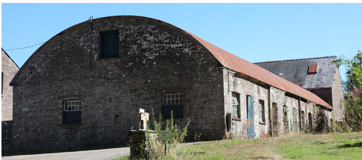
The cow house/dairy at the model farm, Buckland Hall, built with a central feeding passage. It originally appears to have had a double-pile roof of different heights which was later replaced by a single-span arched roof of corrugated iron, the end walls raised and a loft inserted. The loft stored and transferred feedstuff from the adjacent mill. Photo © Sam Hale
