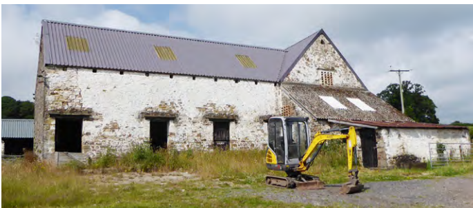
A large early 18th century cow house attached to a large barn with granary of the same date to the east of Llanover (Bloreng Valley and Slopes). Photo © Jeremy Lake
