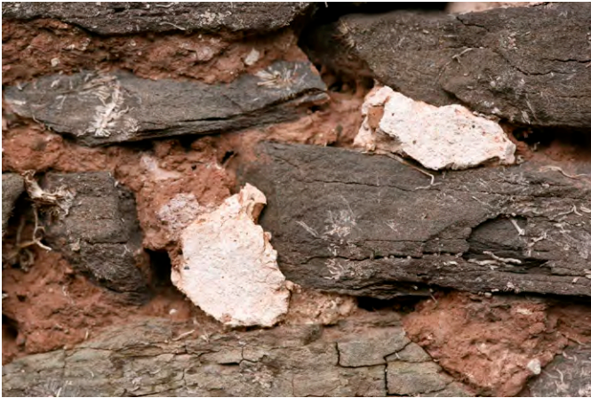
Sandstone laid in an earthen mortar comprising subsoil and quicklime hot mixed with traces of a tight lime plaster/parging coat now much weathered and lost - formerly suggesting the elevation was rendered with a tight coat. Photo © Sam Hale
