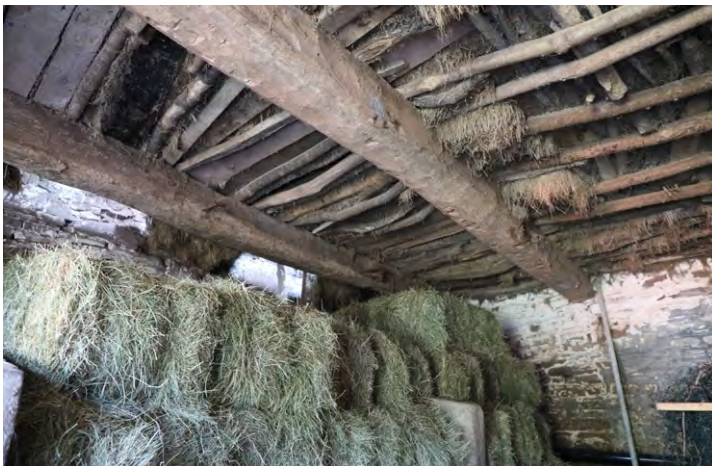
Interior of a Breconshire stable with loft supported on hazel, ash and hawthorn poles. Holes against the wall for dropping hay into the mangers (behind the hay bales). Photo © Sam Hale
