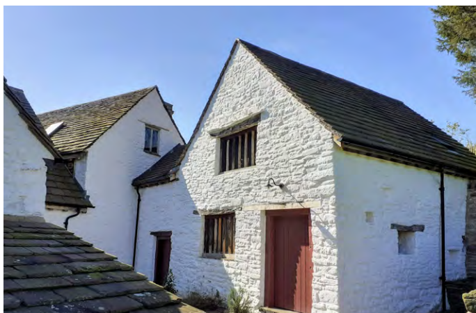
A late 17th century cider house at Llwyn Celyn, Eastern Usk Valley. Photo © Sam Hale
