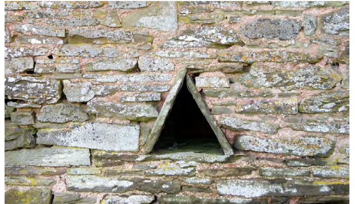
The use of stone tiles to form triangular vents to cattle housing and barns is a common feature. These can be called owl holes, although purpose-made holes for owls are usually set in the gable ends of buildings (usually barns) and can be square in shape. Photo © Sam Hale
