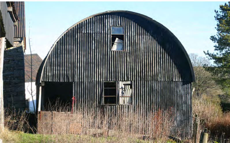
Corrugated iron, the curved profile being typical of roofs from the late 19th to the mid 20th centuries. Photo © Sam Hale
