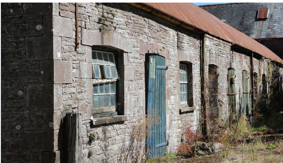
Imported freestone used in the tooled surrounds, sills and quoins of the cow house and dairy range at Buckland Model Farm. Photo © Sam Hale
