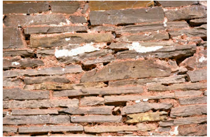
Sandstone laid in an earthen mortar comprising subsoil and quicklime hot mixed with evidence of masonry bee activity and traces of a tight lime plaster/parging coat now much weathered and lost. Photo © Sam Hale
