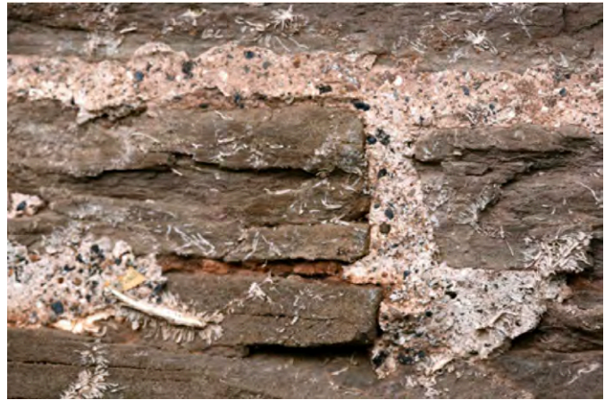
Sandstone laid in an earthen mortar comprising subsoil and quicklime hot mixed with a later 19th century/ early 20th century repair comprising re-pointing finishing mortar comprising lime and aggregate hot mix with pozzolan inclusions of red brick/tile and firing material (coke) from the kiln. Photo © Sam Hale
