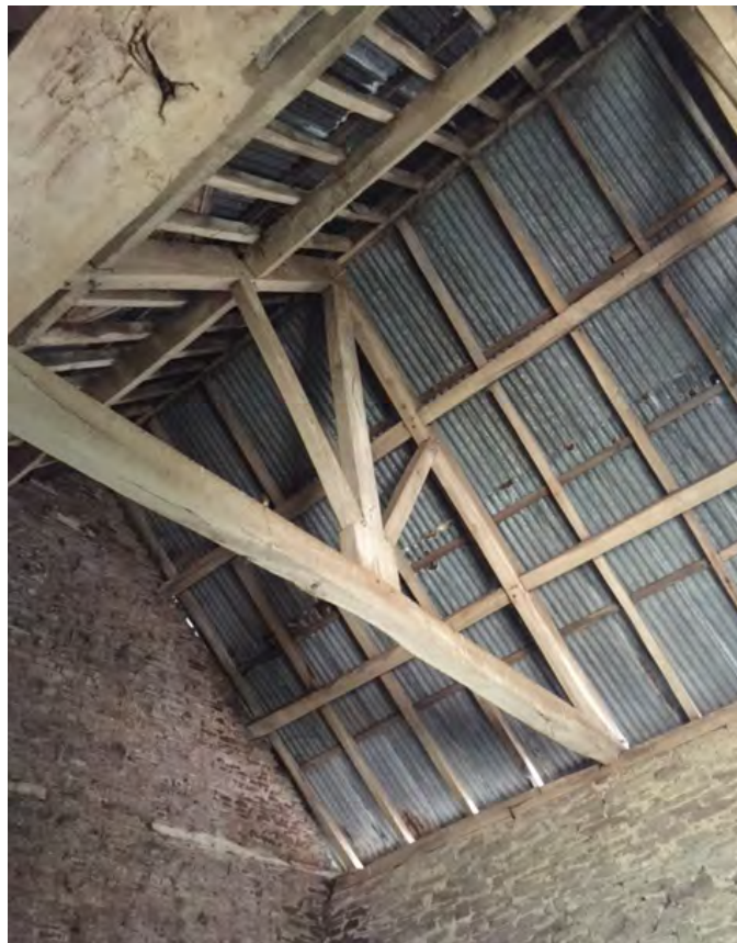
More standardised forms of construction using softwood, as here in this king-post roof truss, becomes widespread in the mid-late 19th century. Photo © Jeremy Lake
