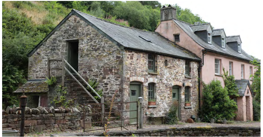
Stables with granary over attached to the house, Priory Mill Farm, Brecon. Photo © Sam Hale
