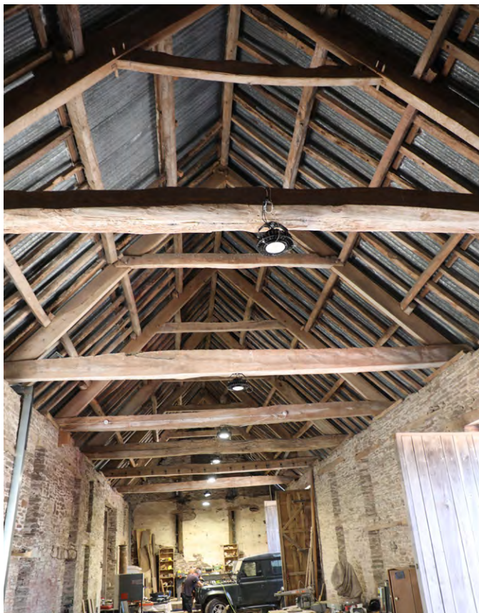
The interior of an early large 18th century 9-bay threshing barn with two threshing floors at Tŷ-Mawr, Llangasty, with its purlins 'trenched' across the backs of the principal rafters, its collars halved and pegged into the principal rafters and the long tie beams made (by using broad axes or adzes) from single tree trunks. Photo © Sam Hale
