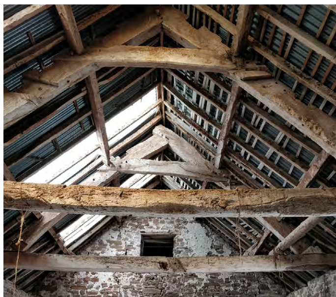
Notches indicate that these roof trusses have been reused in the early 19th century from an earlier building. The lap joints of the near roof-truss are characteristic of reused crucks. The use of wooden pegs to secure ridges and collars declines over the 19th century. Photo © Jeremy Lake
